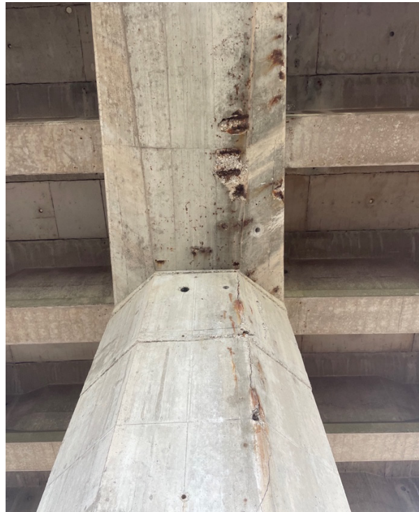
Figure 24: Corrosion and cracks on Pier 5 – Viaduct B.
