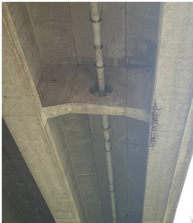
Figure 22: Corrosion on Girder group 1 – Viaduct A.
