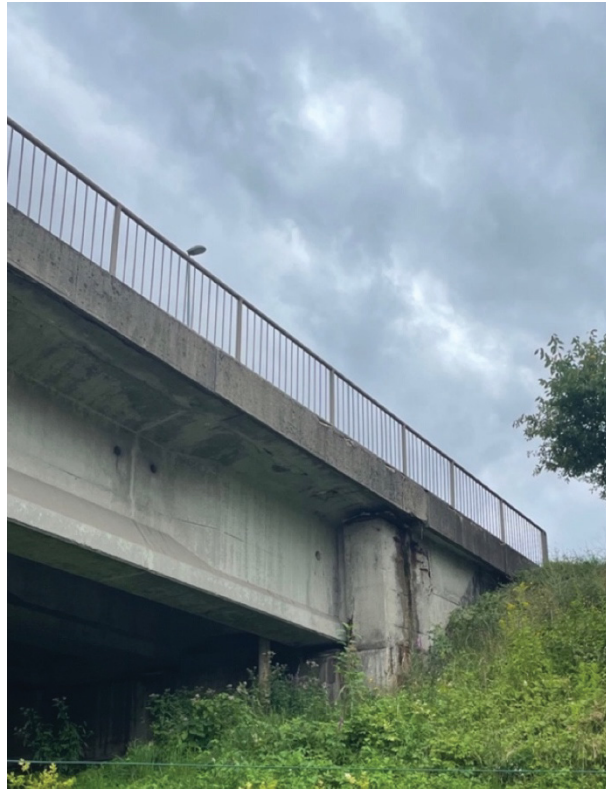
Figure 19: Corrosion on the right Wing – Viaduct A.
