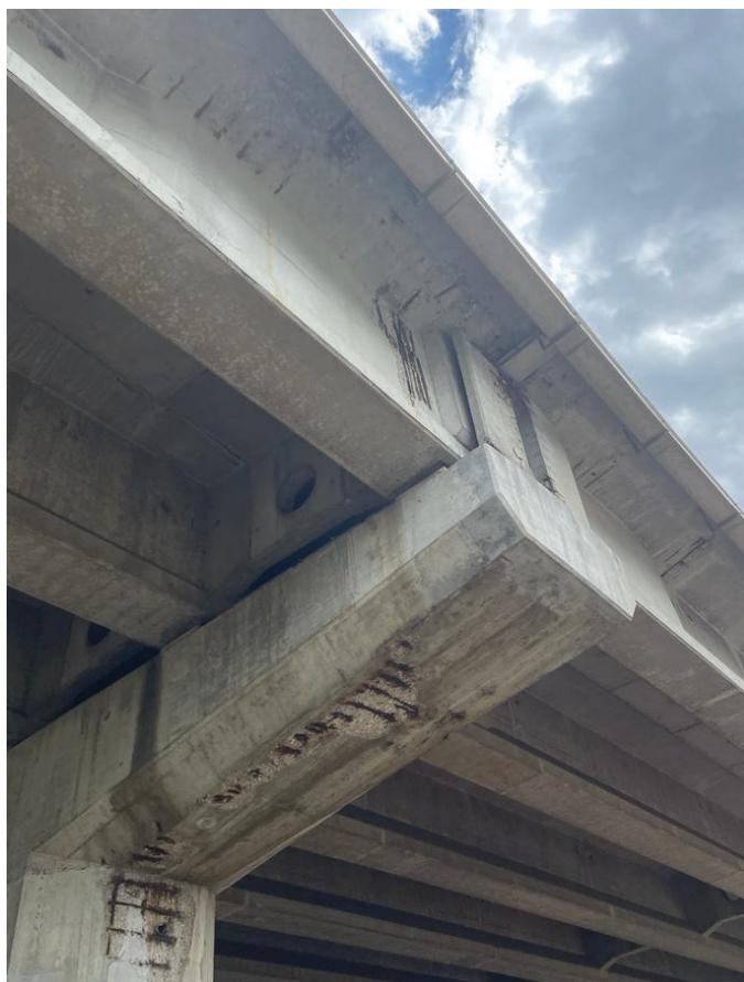
Figure 23: Corrosion on Pier 6 and Girder group 6 – Viaduct B.
