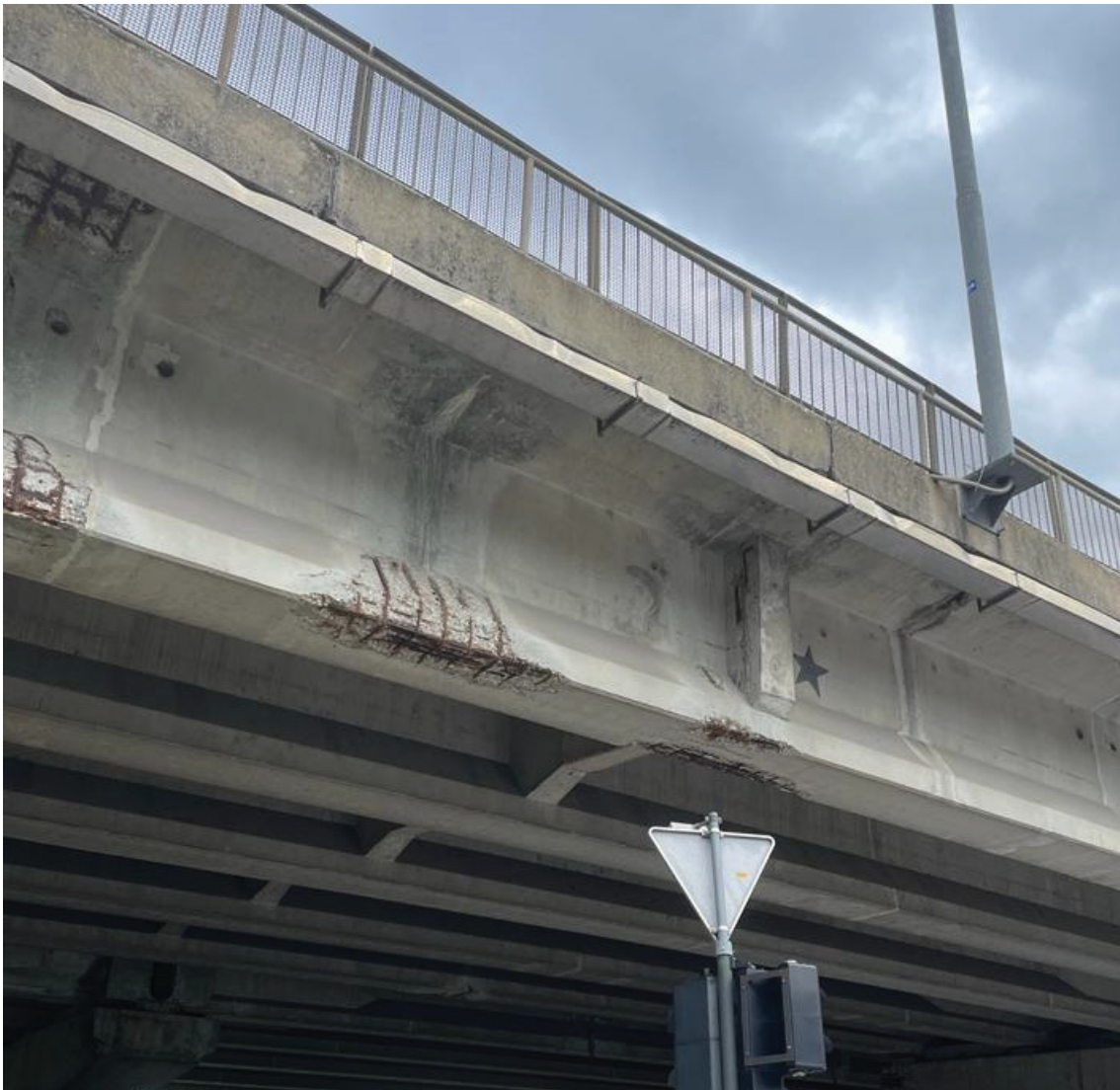
Figure 21: Corrosion on Girder group 3 – Viaduct B.
