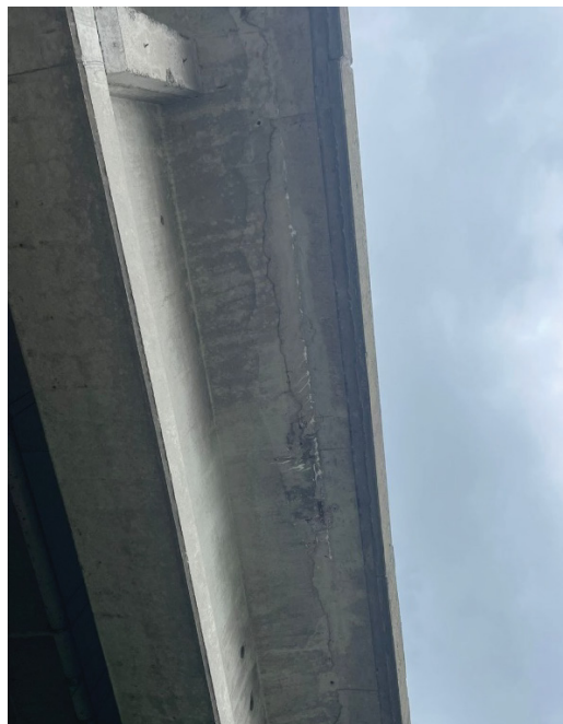
Figure 27: Damage found on the surface below the pedestrian area.
